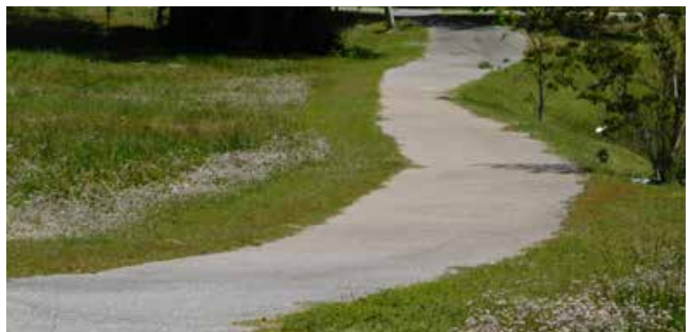
Walk/bike path surface to be repaired and recoated Winter 2019
