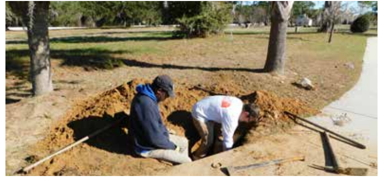
One of a number irrigation leaks
